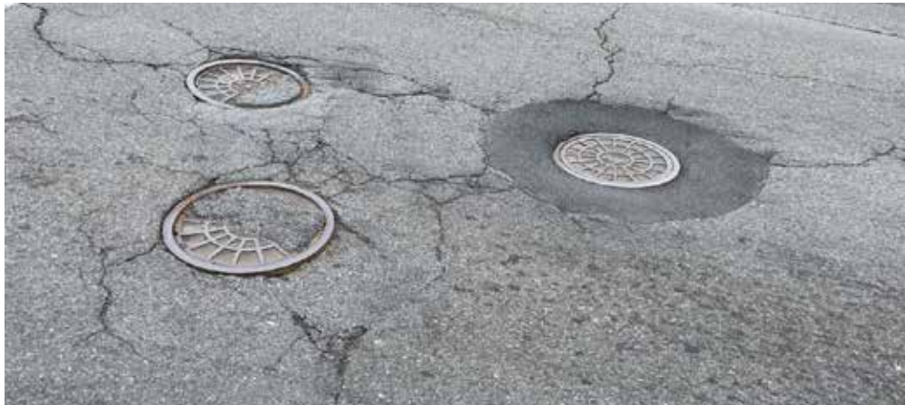
Potholes, craters and uneven surfaces dot Tuckahoe Road, Yonkers. More photos online at YonkersTimes.com
