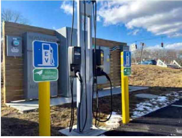
new EV charging stations
