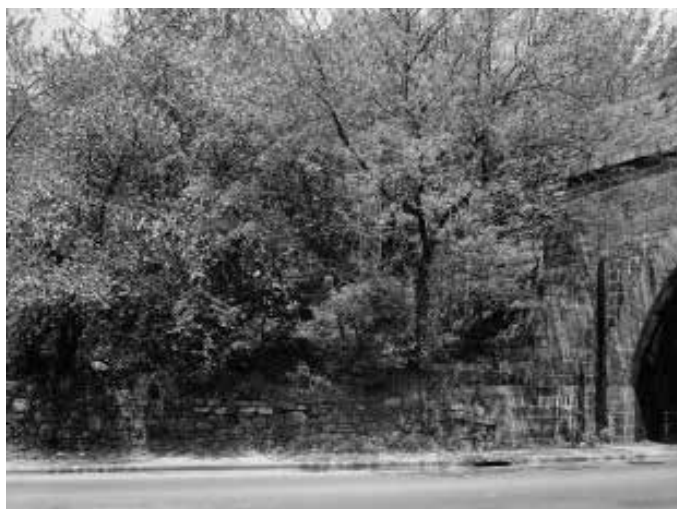
The Nepperhan or Saw Mill River culvert by Nepperhan Avenue in Yonkers.
