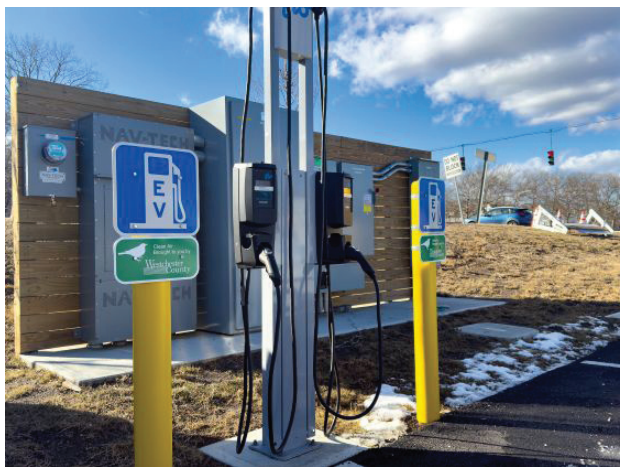
new EV charging stations
